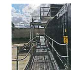
GALVANISED MILD STEEL STAIRS, BALUSTRADE AND PLATFORMS
