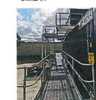
GALVANISED MILD STEEL STAIRS, BALUSTRADE AND PLATFORMS
